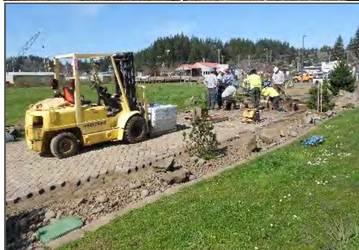
Angell Job Corps brick masonry students lay a brick pathway leading to the Port of Toledo Event Center. Photo courtesy of Brian W. Collins.
