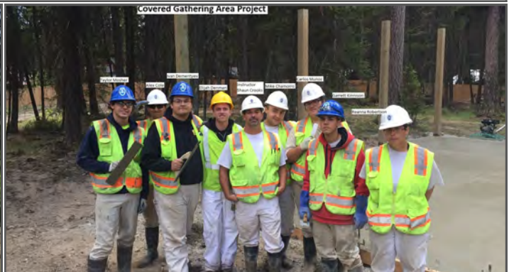
Curlwe Job Corps cement masonry students poured concrete and cut joints for a covered gathering area on Bonaparte National Park for the Tonasket Ranger District on the Colville National Forest August 23-24, 2016.
