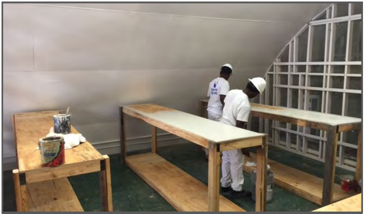
Golconda Job Corps students construct the interior components of the Center's wildland fire cache in Spring 2016. Photo courtesy of Golconda Job Corps.
