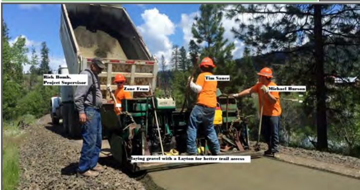
For the past two years, students in Curlwe Job Corps' construction craft laborer trade have worked building the Ferry County Rail Trail that runs on an abandoned railway from the U.S. - Canadian border to Republic, Washington. Photo courtesy of Curlwe Job Corps.
