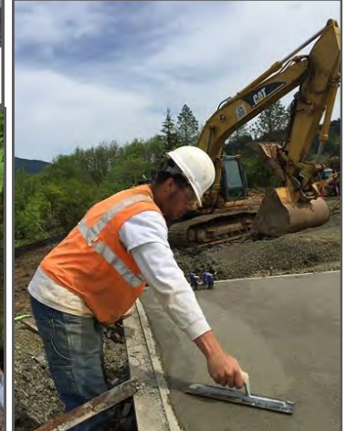
Wolf Creek Job Corps cement masonry student keeps busy on a Work-Based Learning assignment at Dollar Tree. Photo courtesy of Wolf Creek Job Corps.
