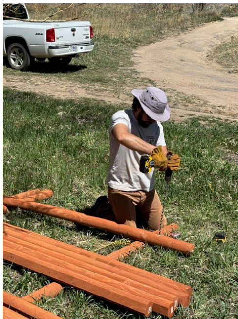
Pikes Peak District employee Daniel Bolderam did all the heavy lifting for us.
